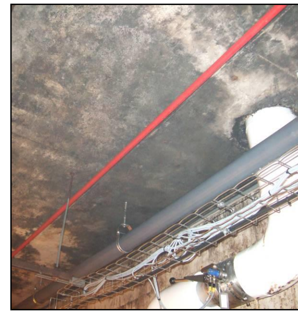
Mold growing on ceiling
