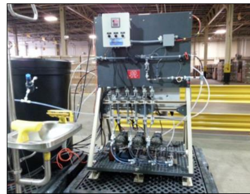
MOS Feed Skid with Free Cl2 Controller and Zone Delivery Pump
