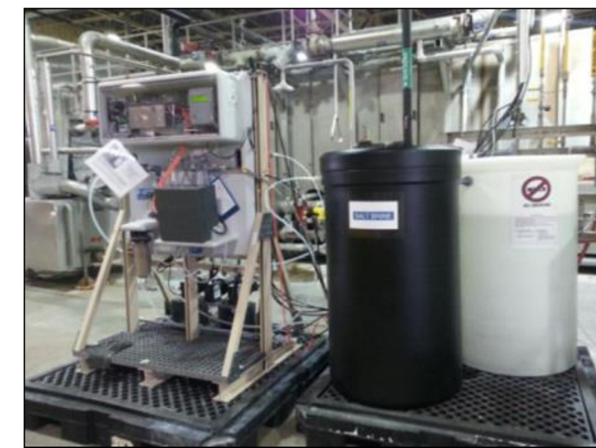
MOS Generation System with Brine and MOS Tank
